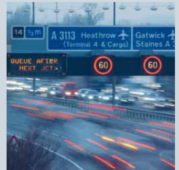
Traffic information and control system
