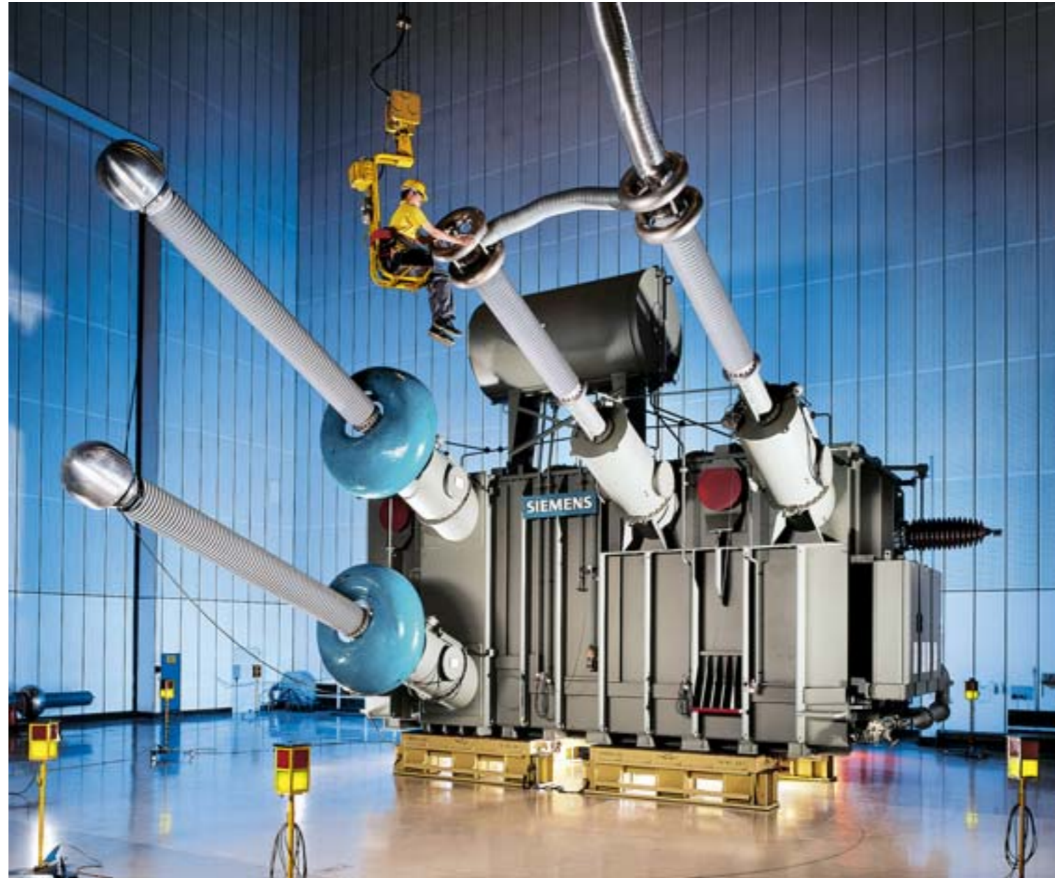
New offshore wind farms (left) will provide a wealth of clean power. High-voltage direct-current transmission insures low-loss transmission over long distances (picture shows a transformer).
